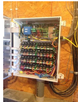
Figure 6. Control system with visible relay cards
