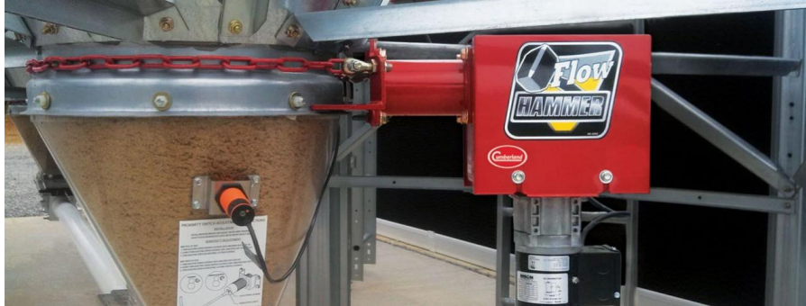
Figure 7. Cumberland Inc. Flow Hammer and proximity sensor mounted to feed bin collar
